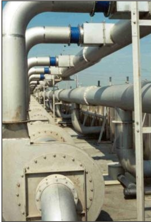
Plate 3.3: Illustration of roof-mounted ductwork to biofilter (operational plant, Italy).
