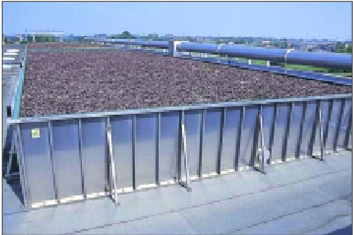
Plate 3.5: Operational roof mounted biofilter (Italian plant).
